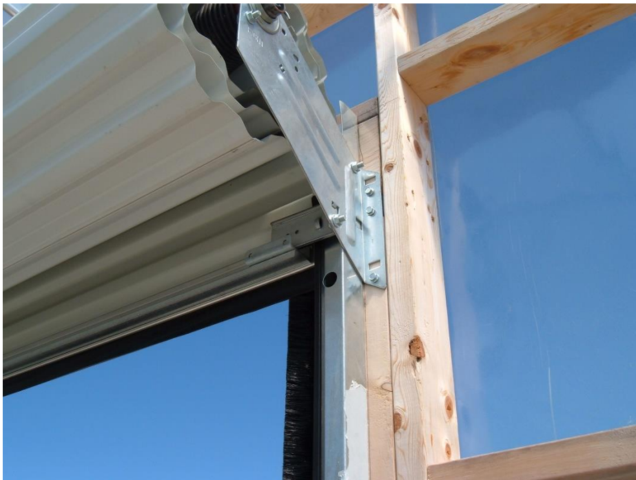
Examples of framing and installation of a roll-up door in the next series of photos
